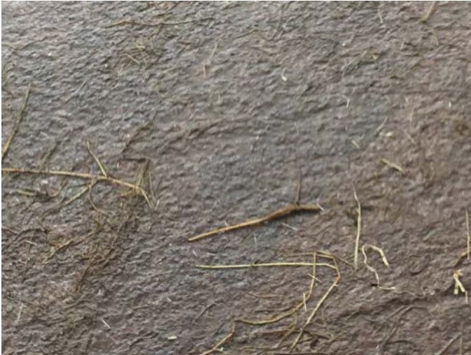
Floors must provide a secure grip, non-slip surface, such as that provided by a heavy brush finish on newly laid concrete
